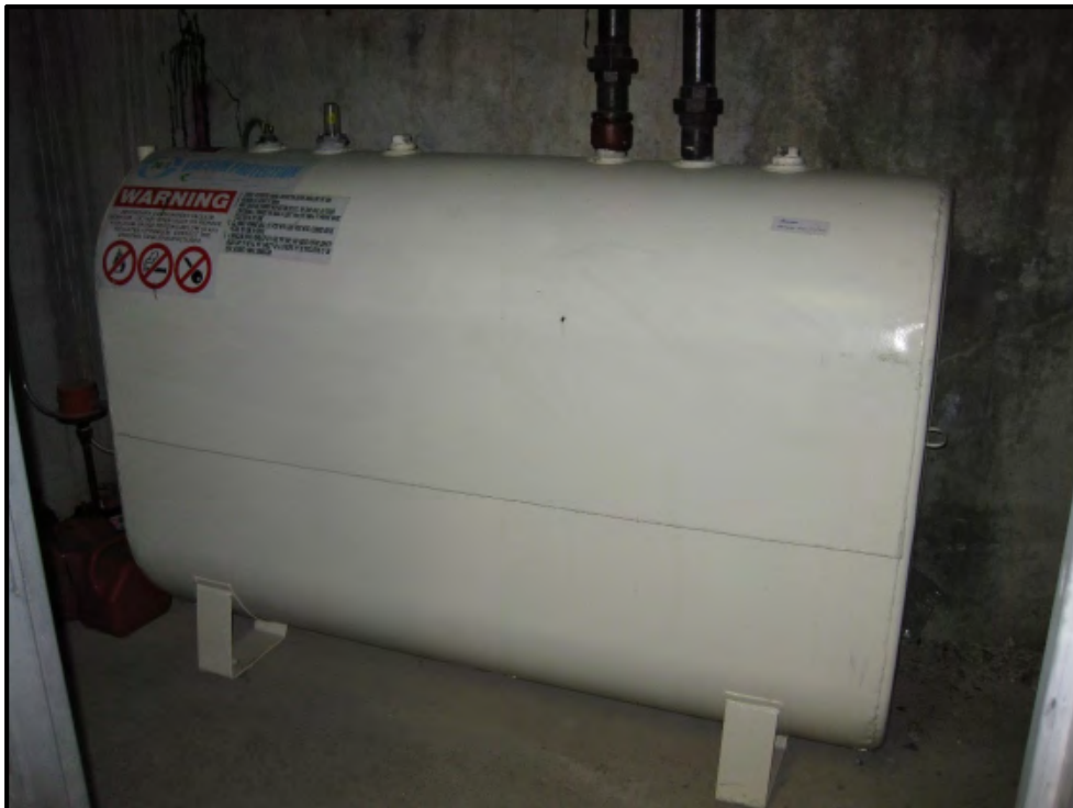
Photograph 12: View of the AST containing diesel for the back-up generator, located in the parking garage at 11 Yorkville Avenue (October 11, 2017).
